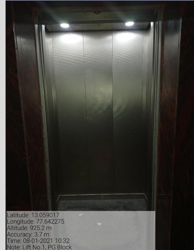
Lift in PG Block
