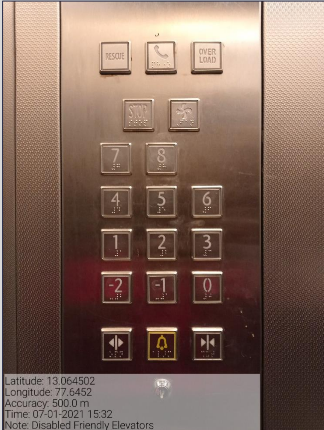
Lift in Admin. Block ( Braille Lift Button)
