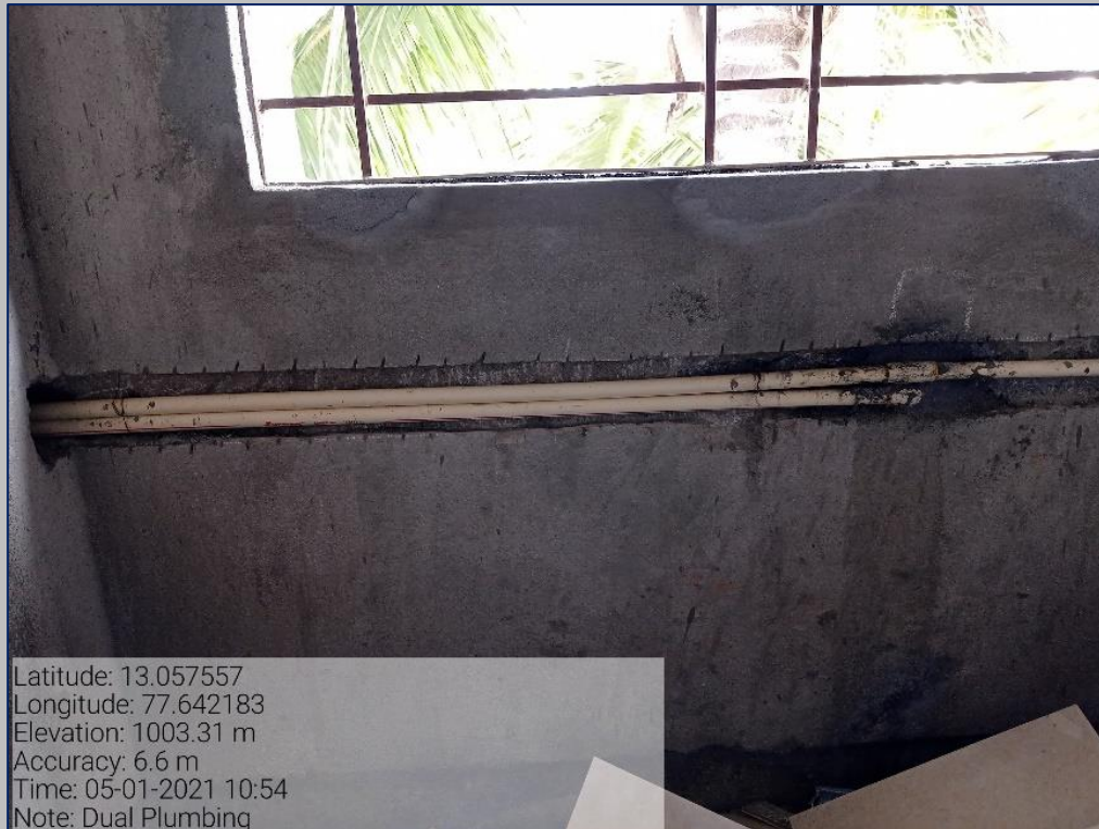
Dual Plumbing for Flushers
