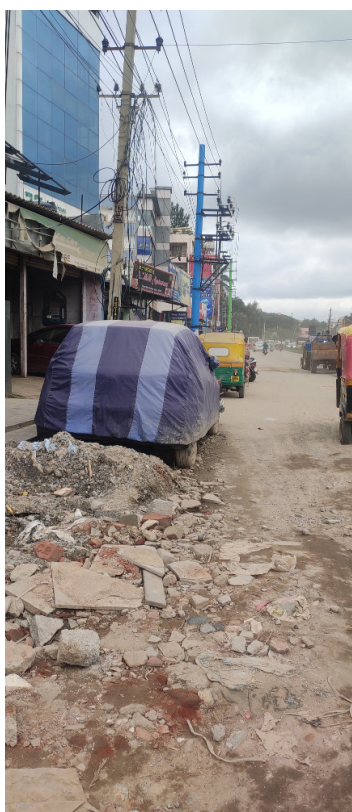
Debris covering the road
