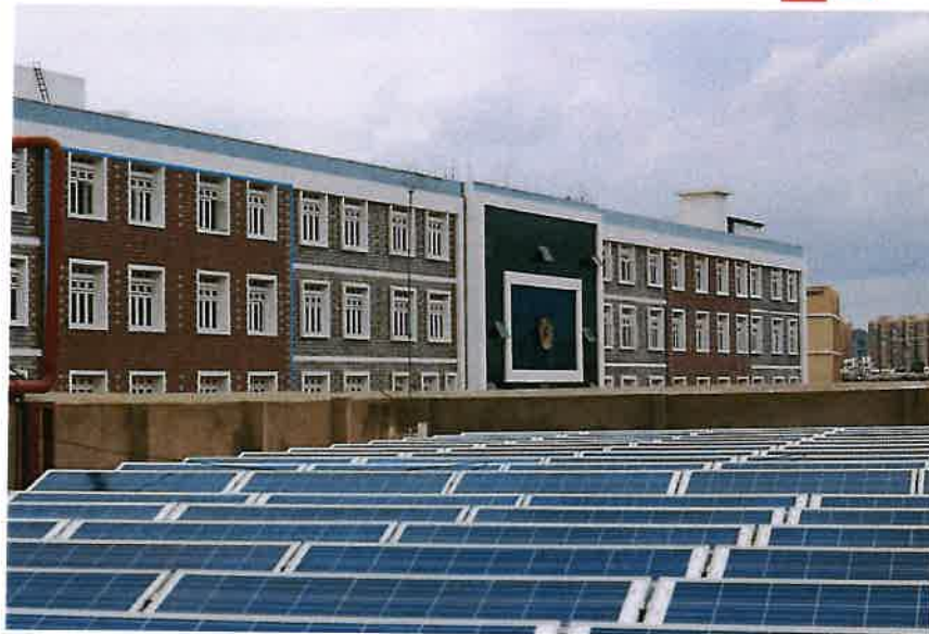
Figure 3: Roof top SPV in campus
