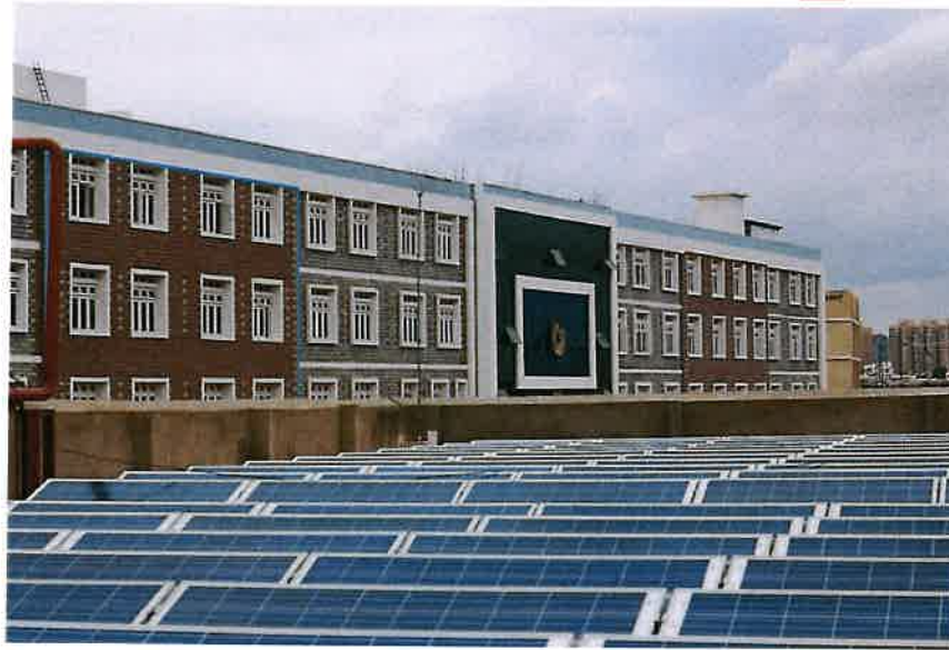
Figure 4: Roof top SPV in campus
