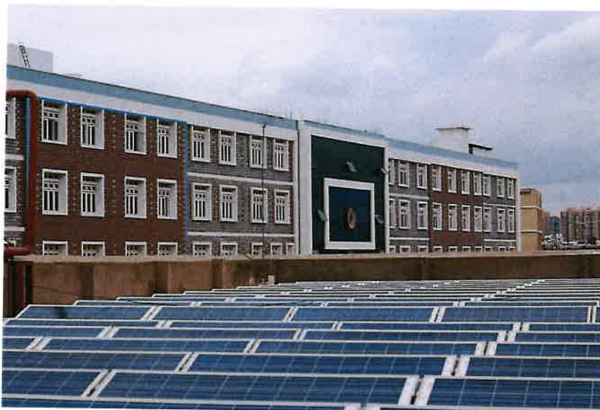
Figure 4: Roof top SPV in campus
