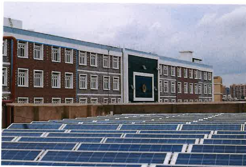
Figure 4: Roof top SPV in campus
