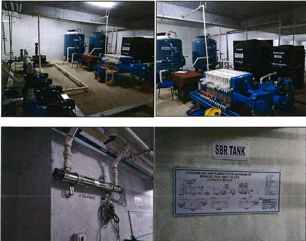
Sewage Treatment Plant
