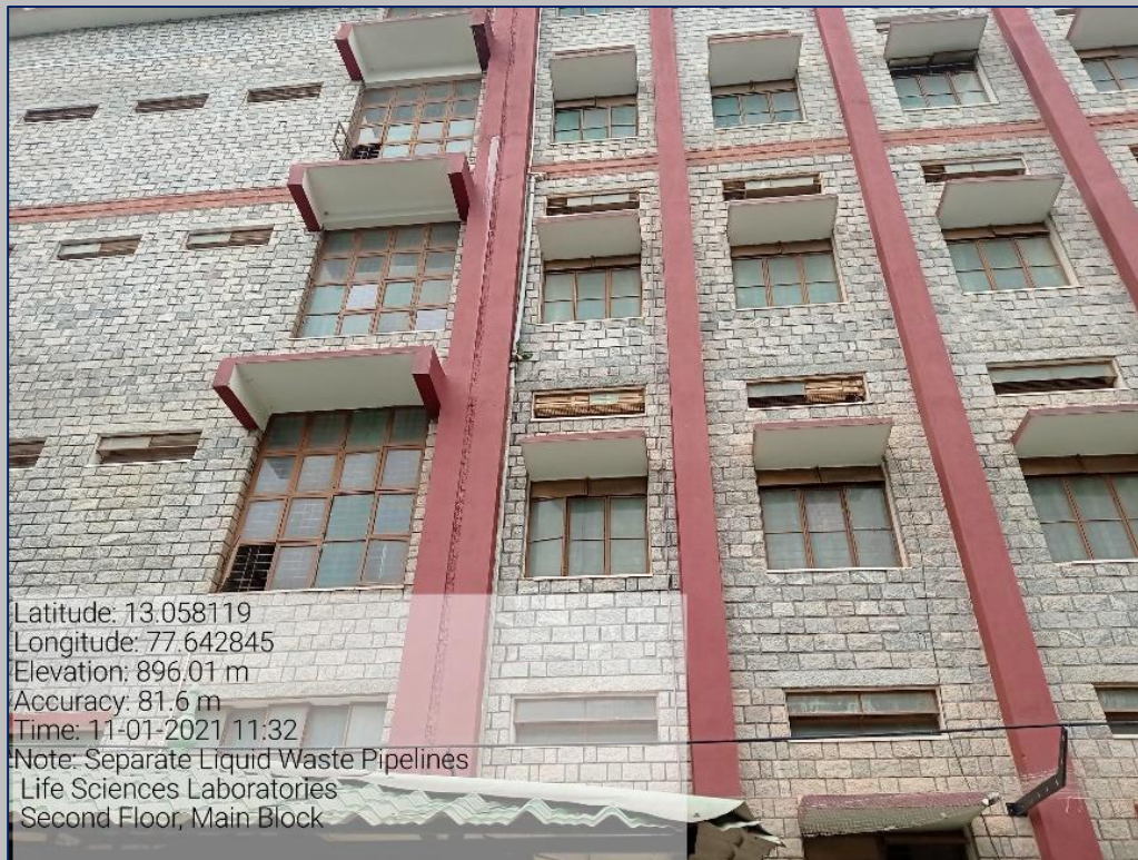
Separate liquid waste pipeline from labs
