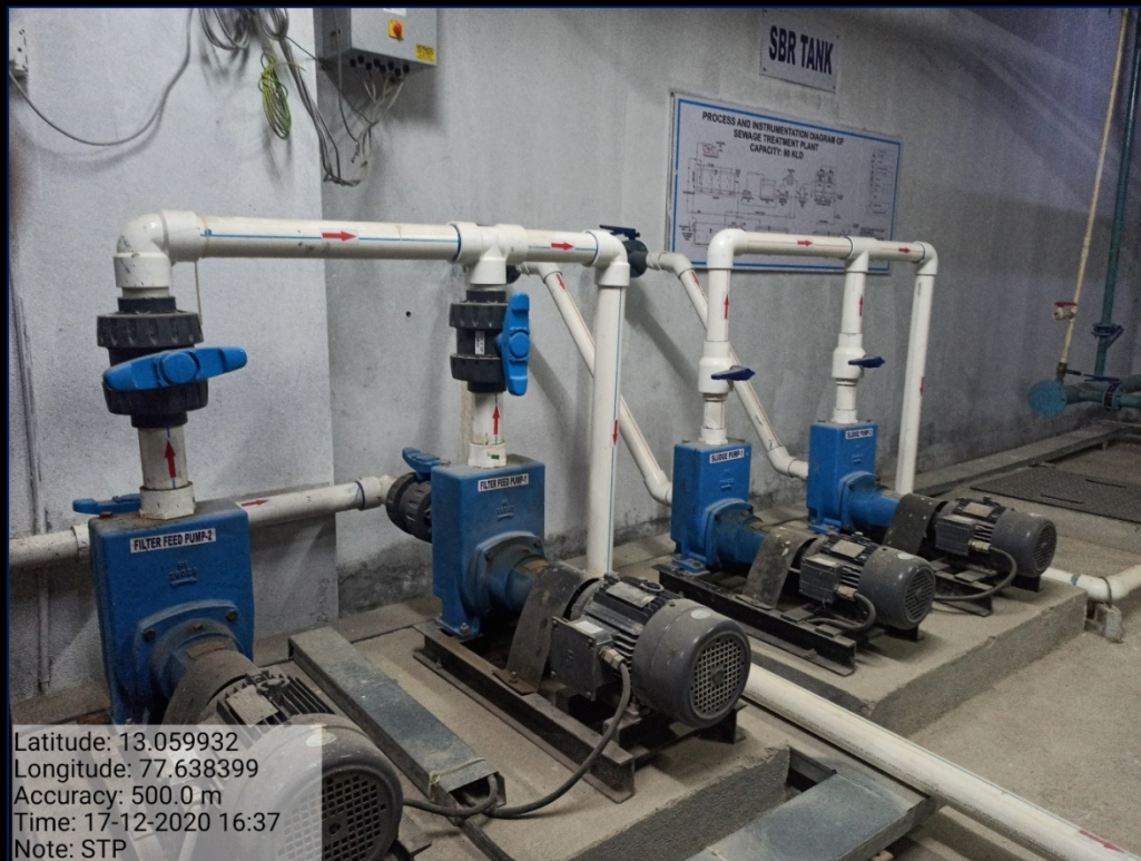
Sequential Batch Reactor (SBR)
